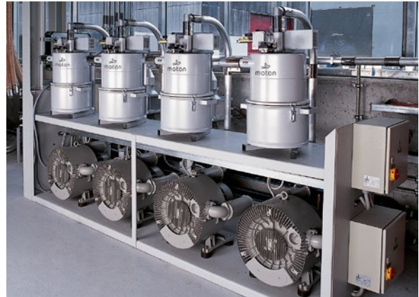
Station d'aspiration centrale
