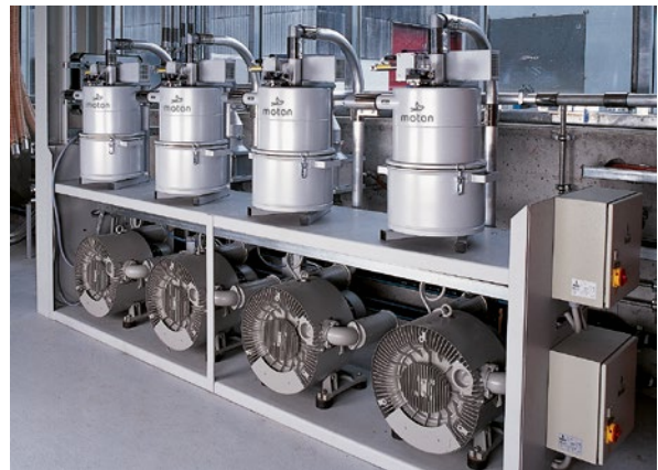
Central vacuum station
