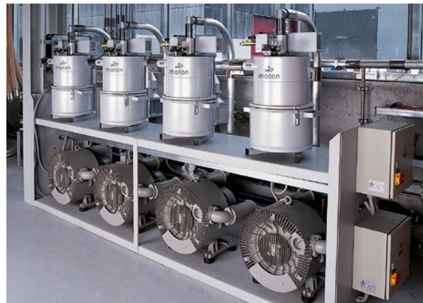
Central vacuum station
